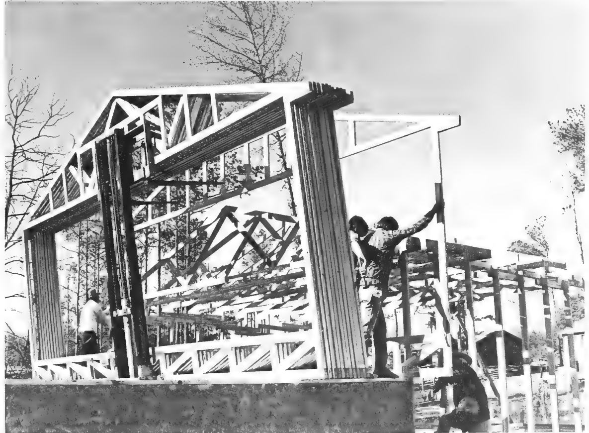
Using the Truss-Frame System, a small crew of laborers can frame up an average house in just a few hours.
